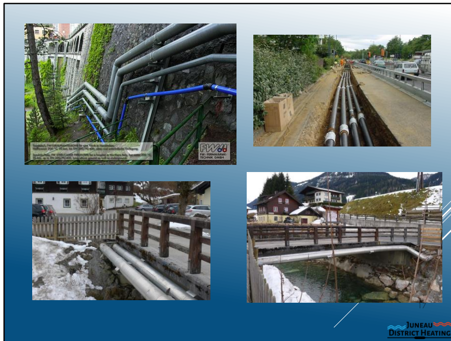
Pipes in Drammen, Norway. Stakeholders of Juneau District Heating, including project leaders, local assembly members, and investors visited Drammen, Norway and took these pictures.
